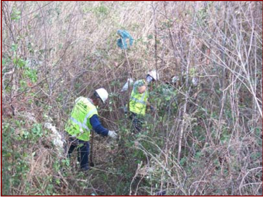
Job No.: 10-21-00, Virginia Department of Transportation @ High Rise Bridge DMS Replacement: foreman, Paul Elliott, Chris Jones, Danny Spears, and George Thompson installing silt fence.
