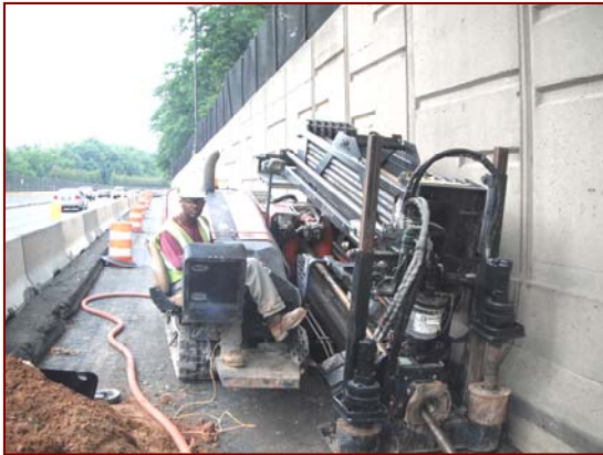
Job No.: 10-10-00, The Lane Construction Company @ I-66 Third Lane Widening: foreman Marvin Edwards installing conduit via directional drilling.
