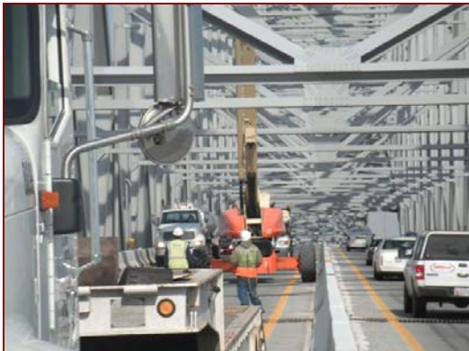
Job No.: 09-19-00, Maryland Transportation Authority @ Navigational Aids at Various Facilities: Superintendent James Hartwell along with crew members Billy Burton IV and Kyle Wratten removing and installing aerial beacons at the Francis Scott Key Bridge in Baltimore City, MD.
