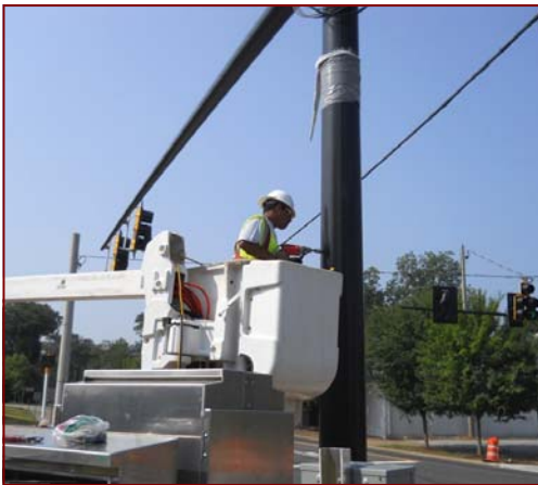
Job No.: 10-18-00, Coweta County, GA @ Traffic Signal Upgrade: foreman Martin Zuno installing a pedestrian traffic signal head.
