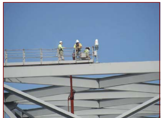
Job No.: 09-19-00, Maryland Transportation Authority @ Navigational Aids at Various Facilities: Superintendent James Hartwell along with crew members Billy Burton IV and Kyle Wratten removing and installing aerial beacons at the Francis Scott Key Bridge in Baltimore City, MD.
