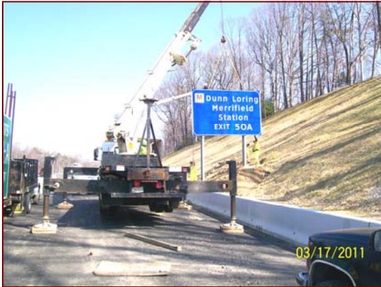
Job No.: 06-16-00, Fluor/Lane, LLC @ I-495 HOT Lanes: foreman Richard Henderson and crew installing ground mount posts & signs.
