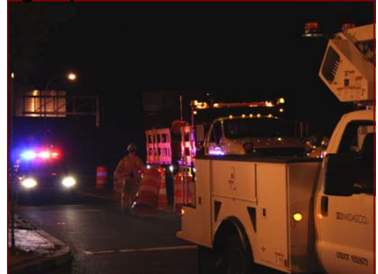
Job No.: 10-25-00, Delaware Department of Transportation @ Statewide LED Relamping: crews setting up maintenance of traffic.
