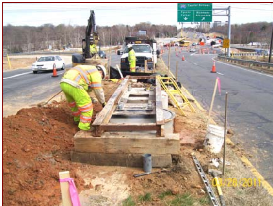
Job No.: 06-16-00, Fluor/Lane, LLC @ I-495 HOT Lanes: foreman Richard Henderson and crew working on sign foundations.
