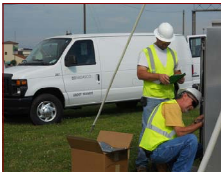
← Job No.: 10-04-00, City of Hickory, NC @ Traffic Signal System Upgrade: Superintendent Ron Johnson and Technical Manager Jeff Hensley are installing new traffic signal controllers.
