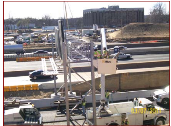
Job No.: 06-16-00, Fluor/Lane, LLC @ I-495 HOT Lanes: foreman Denis Zelaya and crew installing an overhead sign structure truss.
