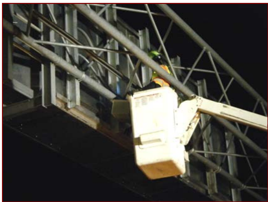
Job No.: 10-15-00, North Carolina Department of Transportation @ Division 10, DMS Replacement: Kevin Ashbey, Jr. working on conduits for dynamic message sign.
