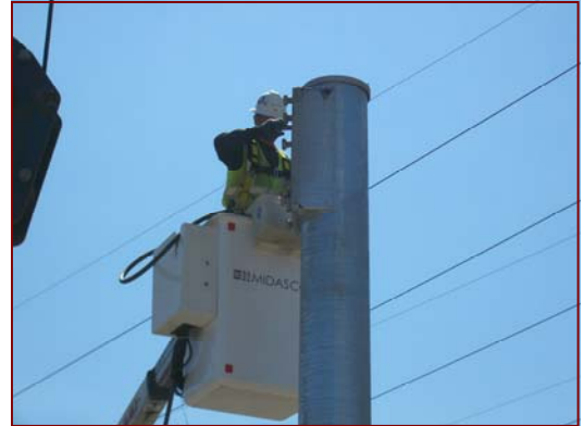
Job No.: 07-07-00, Virginia Department of Transportation Eastern Regional Traffic Signal Maintenance: Robert Bussey preparing to install a traffic signal pole.
