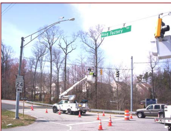
Job No.: 08-06-00, Maryland State Highway Administration @ Signal Systemization— Districts 3,4, &5: foreman Rick Knowles along with crew members, Angel Osorio, Otto Lopez, & Sidney Garbutt upgrading traffic signals from incandescent to LED in Harford County.
