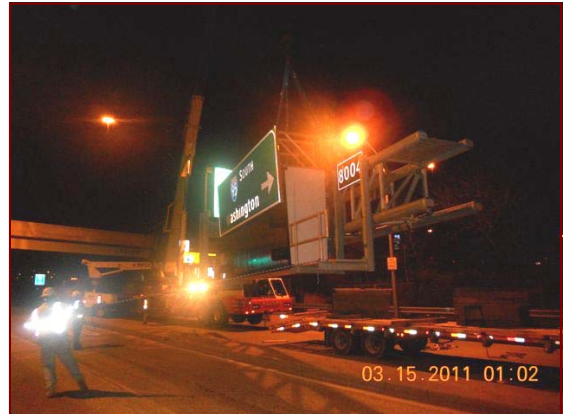
Job No.: 09-10-00, Maryland Transportation Authority @ Signing North of Fort McHenry Tunnel: subcontractor, RN'G Construction, installing a sign structure.
