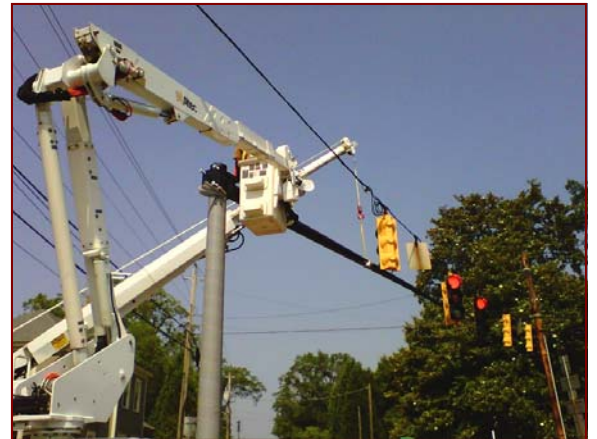
Job No.: 10-18-00, Coweta County, GA @ Traffic Signal Upgrade: foreman Baldemar Avalos and Foreman Martin Zuno installing mast arm signal poles.
