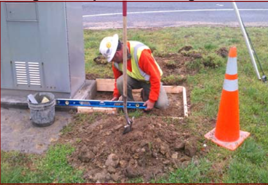
Job No.: 07-07-00, Virginia Department of Transportation Eastern Regional Traffic Signal Maintenance: Robert Bussey leveling a cabinet foundation form.
