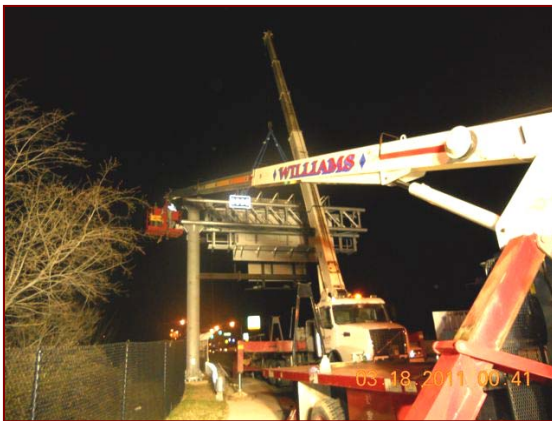
Job No.: 09-10-00, Maryland Transportation Authority @ Signing North of Fort McHenry Tunnel: subcontractor, RN'G Construction, installing a cantilever sign structure.
