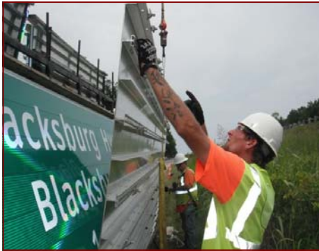
Job No.: 10-23-00, South Carolina Department of Transportation @ Spartanburg and Cherokee Counties Signing: Foreman Danial Weber unloading extruded panel sign for installation.
