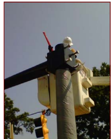
Job No. 10-18-00: Coweta County, Georgia @ Traffic Signal Upgrades: Foreman Baldemar Avalos and Foreman Martin Zuno installing signal pole arms.
