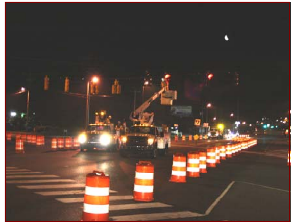
Job No.: 10-25-00, Delaware Department of Transportation @ Statewide LED Relamping: changing from incandescent to LED lamps on traffic signal heads.
