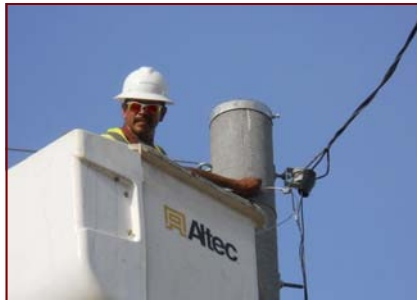
Job No.: 10-22-00, Georgia Department of Transportation @ Bartow County Signal Intersection: installing antenna for wireless system.
