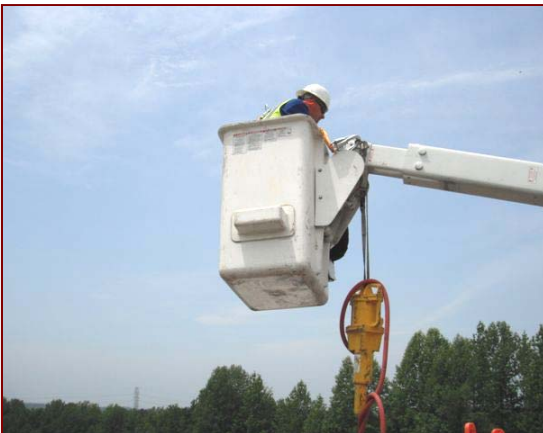
Job No.: 10-23-00 South Carolina Department of Transportation @ Spartanburg and Cherokee Counties Signing: operator Christopher Land installing U-channel sign posts.
