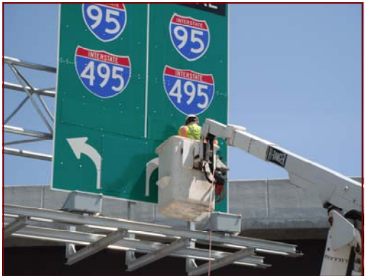
Job No.: 07-15-00, Corman/Kiewit Joint Venture @ Telegraph Road Interchange: Helmer Andrader in the bucket truck installing sign overlays on 95/495.
