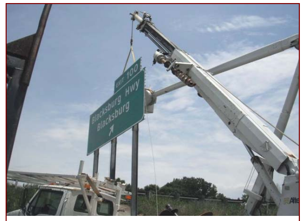
Job No.: 10-23-00 South Carolina Department of Transportation @ Spartanburg and Cherokee Counties Signing: foreman Daniel Weber along with operator John Kirkland installing an extruded panel sign.
