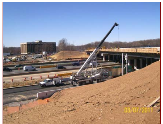
Job No.: 06-16-00, Fluor/Lane, LLC @ I-495 HOT Lanes: foreman Denis Zelaya and crew installing an overhead sign structure truss.
