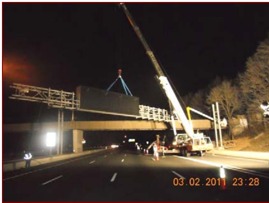
Job No.: 09-10-00, Maryland Transportation Authority @ Signing North of Fort McHenry Tunnel: subcontractor, RN'G Construction, installing dynamic message signs.
