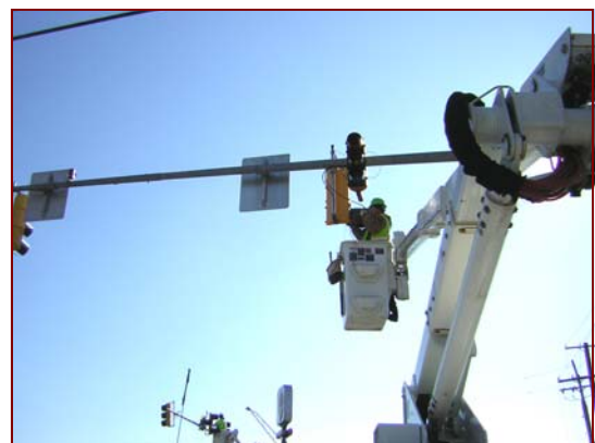
Job No.: 08-06-00, Maryland State Highway Administration @ Signal Systemization-Districts 3,4, &5: foreman Rick Knowles along with crew members, Angel Osorio, Otto Lopez, & Sidney Garbutt upgrading traffic signals from incandescent to LED in Harford County.
