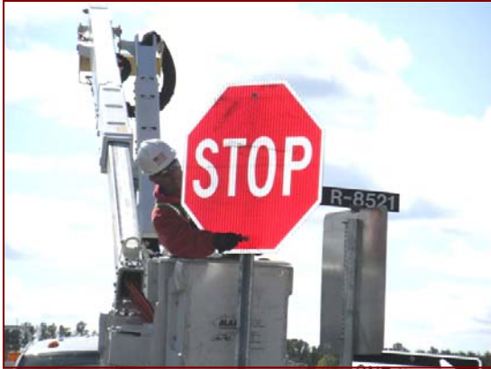
Job No.: 10-23-00, South Carolina Department of Transportation @ Spartanburg and Cherokee Cos Signing: Chris Land changing out a stop sign.
