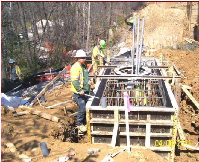
Job No.: 06-16-00, Fluor/Lane, LLC, a joint venture: Crews preparing to pour concrete for a sign structure foundation.
