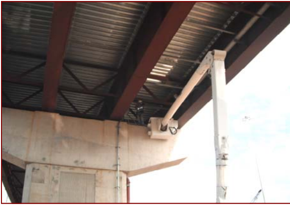
Job No.: 07-15-00, CK Constructors, a joint venture of Corman Construction and Kiewit Corporation: crews pulling fiber optic cable under a bridge.
