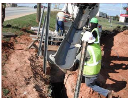
Job No: 10-23-00, South Carolina Department of Transportation @ Spartanburg and Cherokee Cos Signing: Foreman Fred Garrett and Jeremiah Delehanty pouring a foundation for an overhead sign structure.
