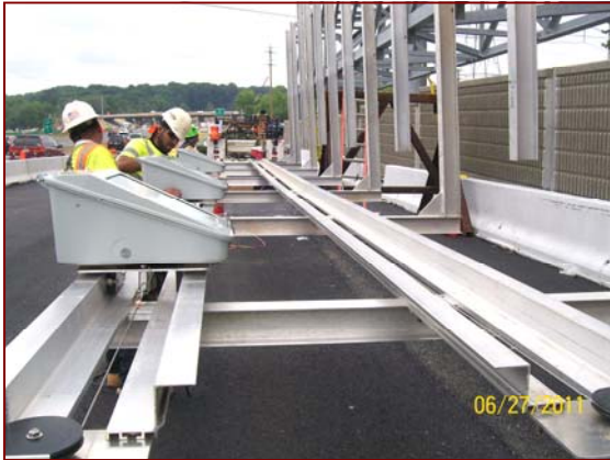
Job No.: 06-16-00, Fluor/Lane, LLC, a joint venture: crews installing Lumitrak sign lighting system on a sign structure.
