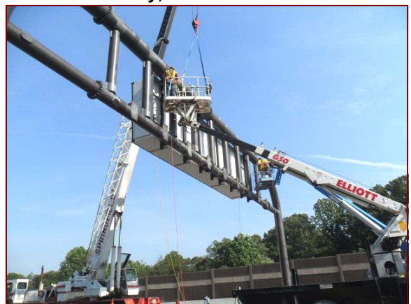
Job No.: 07-14-00: A Joint Venture of Shirley Contracting Company, Facchina Construction Company, Clark Construction and Trumbull Corporation @ ICC, Contract C: Superintendent John Mallinson along with Foreman Elmer Sandoval and crew installing a Variable Message Sign.
