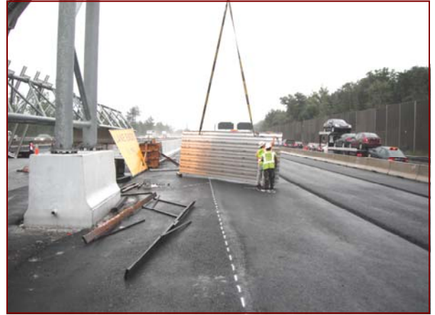
Job No.: 07-15-00, CK Constructors, a joint venture of Corman Construction and Kiewit Corporation: crews preassembling an overhead sign structure.
