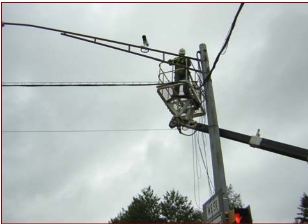
Job No.: 09-06-00, Maryland State Highway Administration @ Inst/Recon Traffic Signals Districts 3,4, &5: Superintendent Rick Knowles and crew member Shawn Williamson pulling traffic cable.
