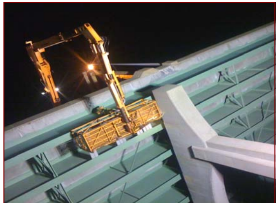
Job No.: Job No.: 10-21-00, Virginia Department of Transportation @ High Rise Bridge DMS Replacement: Superintendent David Floyd installing steel beam that will eventually support a new sign structure.
