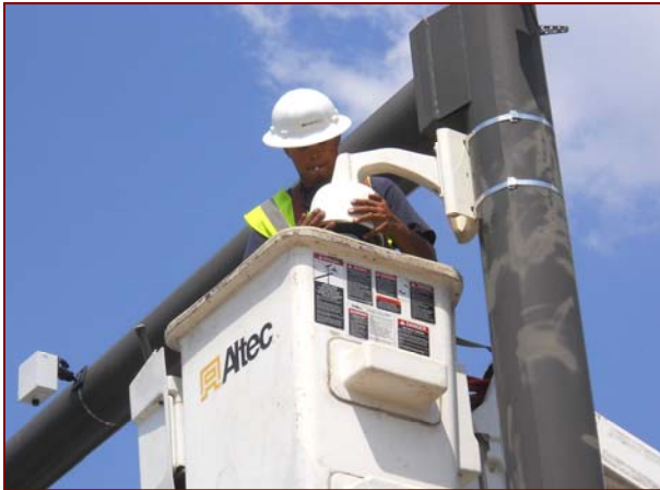
Job No.: 10-24-00-00, City of Alpharetta, Georgia @ Windward Parkway ATMS: Laborer Jose Pimentel is installing a CCTV camera.
