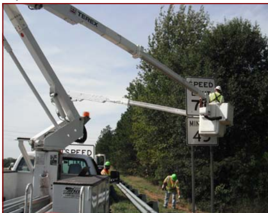
Job No: 10-23-00, South Carolina Department of Transportation @ Spartanburg and Cherokee Cos Signing: Foreman, Fred Garrett and Chris Land installing speed limit signs.
