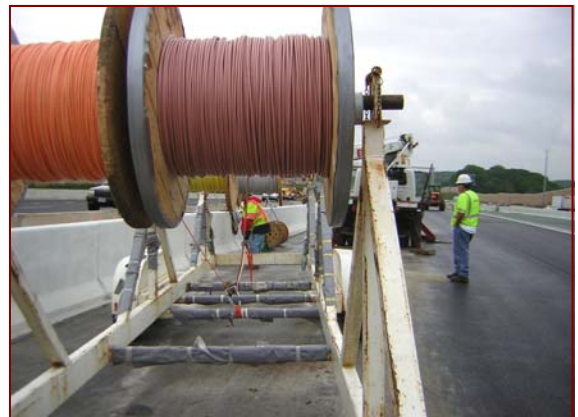
Job No.: 07-13-00, Cherry Hill @ I-95 XLT I-895 to Chesaco: Superintendents Rick Knowles and James Hartwell along with crew leader Sidney Garbutt and crew member Wilman Carballo pulling cable in barrier wall for sign lighting.
