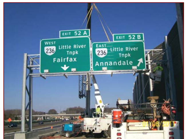
Job No.: 06-16-00, Fluor/Lane, LLC, a joint venture: crews installing a sign structure truss and signs.
