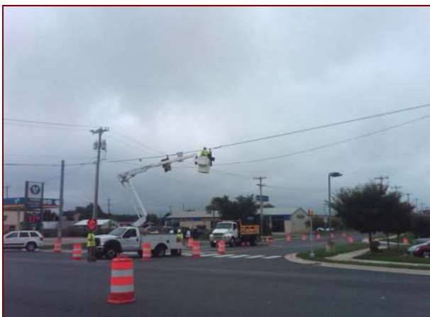
Job No.: 10-25-00, Delaware Department of Transportation @ Statewide LED Relamping: crews changing from incandescent to LED lamps on traffic signal heads.
