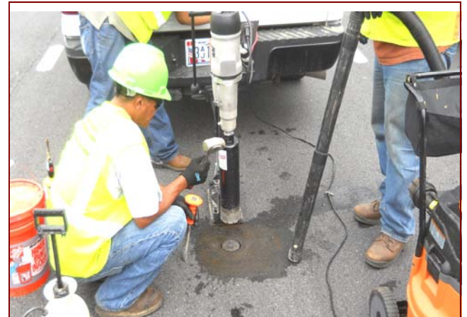
Job No.: 10-24-00-00, City of Alpharetta, Georgia @ Windward Parkway ATMS: Laborer Santos Fajarda is preparing to remove the cored asphalt in order to install a traffic sensor.
