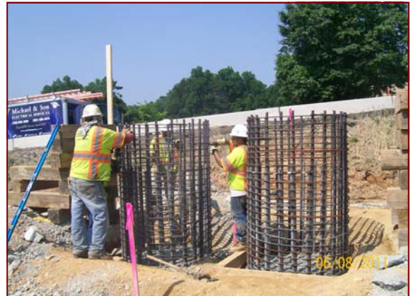
Job No.: 06-16-00, Fluor/Lane, LLC, a joint venture: crews preparing concrete footers for sign foundations.
