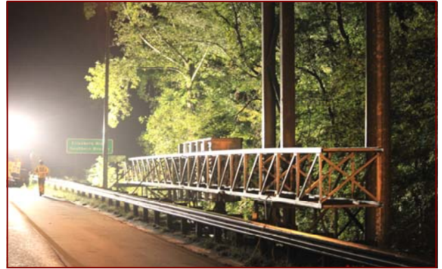
Job No.: 10-21-00: Foremen Stacy White and Paul Elliott's crew installing a sign structure truss and Variable Message Sign.
