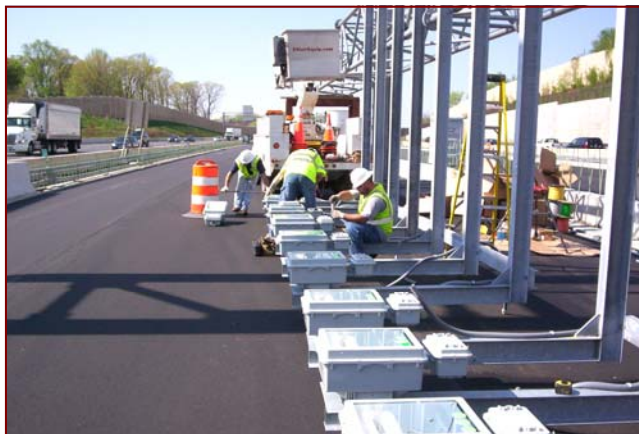
Job No.: 07-13-00, Cherry Hill @ I-95 XLT I-895 to Chesaco: Superintendent Rick Knowles, Foreman Robert Bauman along with crew leader Sidney Garbutt and crew members building sign lighting for overhead sign structures.
