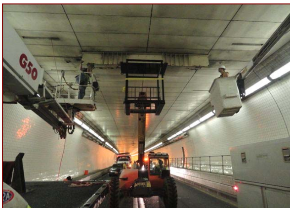
Job No.: 09-13-00, Maryland Department of Transportation @ Fort McHenry Tunnel Sign System update: crews removing and replacing lane control signs.
