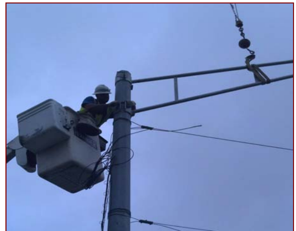
Job No.: 09-06-00, Maryland State Highway Administration @ Inst/Recon Traffic Signals Districts 3,4, &5: Superintendent Rick Knowles and crew member Shawn Williamson pulling traffic cable.
